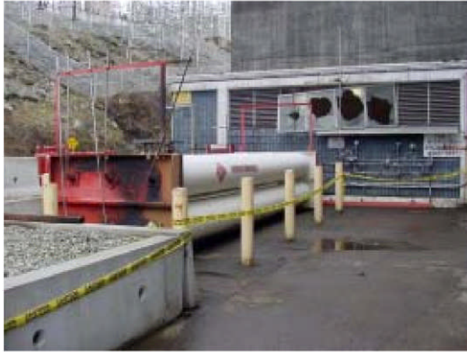
Figure 3. A burn pattern on the hydrogen tube six pack west frame. Note the vent pipe is missing from tube No. 6.
